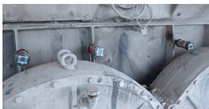
Lubrication of a raw mill
