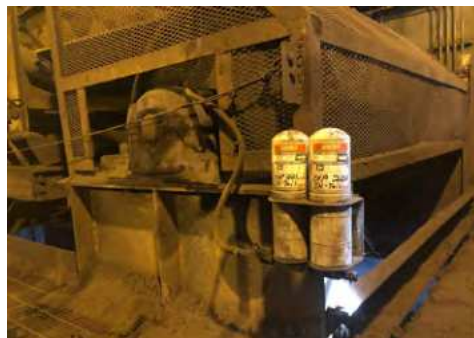
Lubrication on a conveyor
