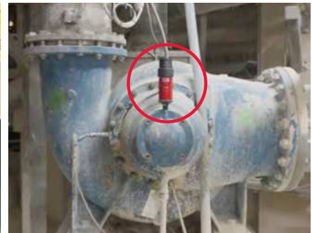
Bearing lubrication on a pump
