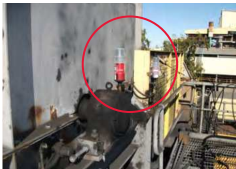
Lubrication systems on a conveyor
