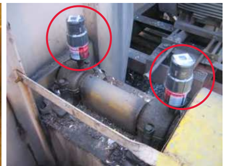
Lubrication of a fan drive shaft bearing
