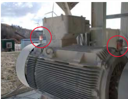
Motor lubrication on a vibrating screen
