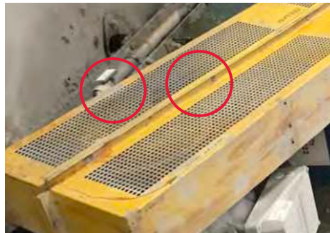
Lubrication of pillow block bearing on a fan
