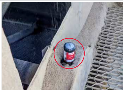
Lubrication of pillow block bearing on grit and sand screen
