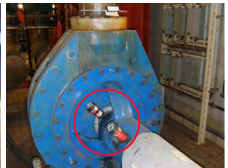
Drive shaft lubrication on a pump
