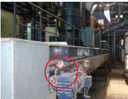
Flange bearing lubrication on a conveyor
