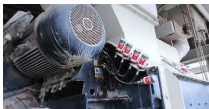
Lubrication of mixing shafts and mixer flaps
