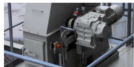
Roller bearing lubrication on a filler elevator
